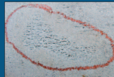
Figure 4. Typical stress corrosion cracking detected with an in-line inspection tool.
